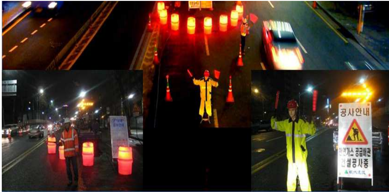
Flagmen and robotic flagmen in front of the construction site. Self-emitting traffic safety signs on the road.
